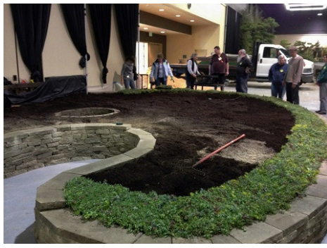
Finally, the walls are built, the mulch has been spread and the sedum border tiles are in place.
